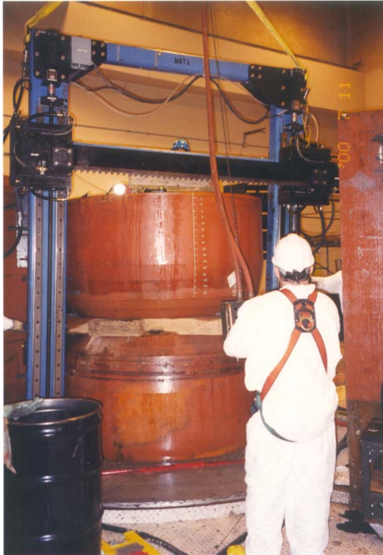
Fig 8 – Photo of the MOTA Reciprocating Machine Tool mounted on the upper pole yoke immediately prior to start of cutting.
