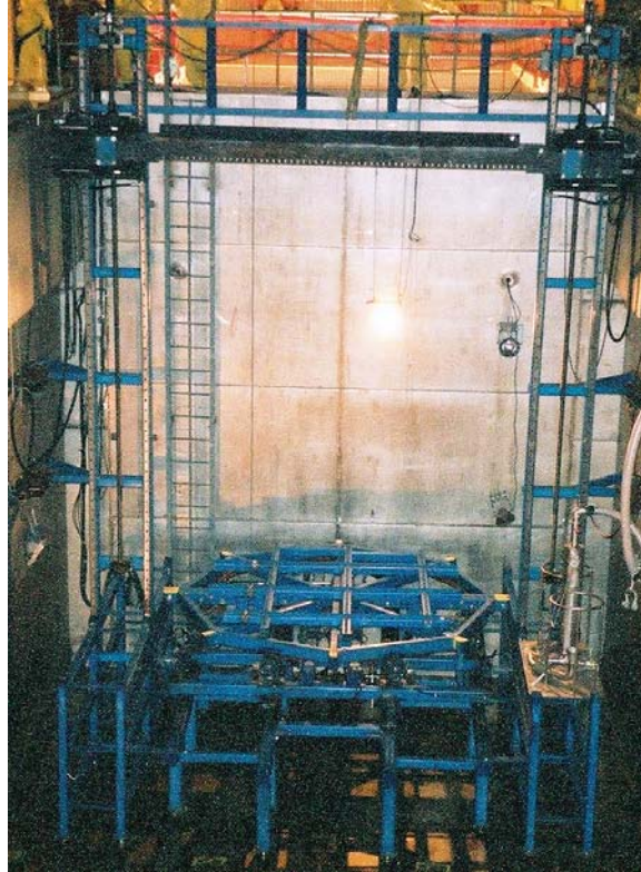
Fig. 2. RMT and associated work platform prior to cavity flood up.
